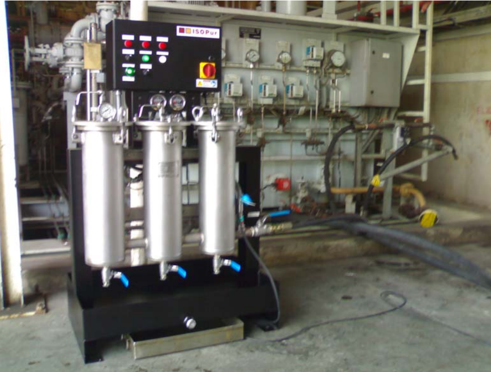
Photo 1 – Varnish Purification System
